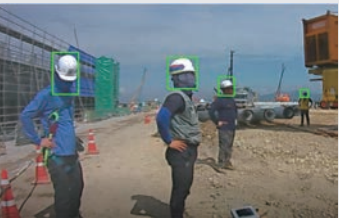
VISION AI-based on-site safety monitoring
